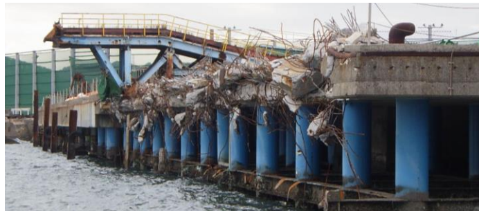
Pier struck and damaged by a vessel drifting in a typhoon
