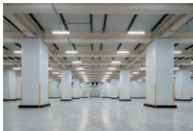
► Multi-tenant logistics facility with fully adjustable temperature control (-25°C to +10°C)
