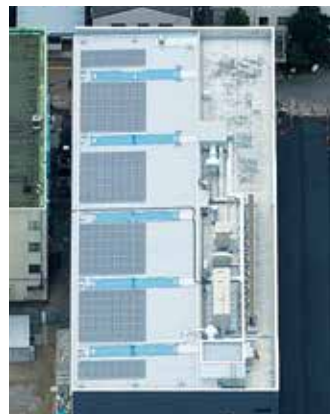
Rooftop solar panels
