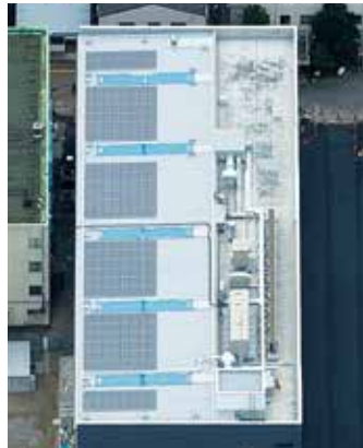
Rooftop solar panels
