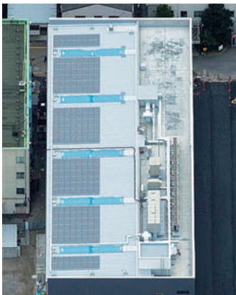
Rooftop solar panels
