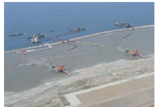
TOA's "Plug Magic" dredging method (see page 14 for details) was adopted in order to maximize the recycling of dredged soft materials
