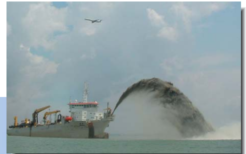
KAISHUU has been adopted to reclamation projects in Asian and Arabic countries to develop new man-made lands for residential lots.
